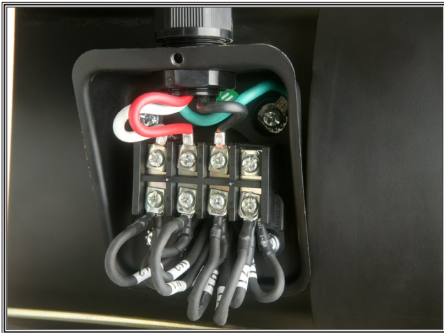
Figure 79. W1762 motor junction box, 220V 3-phase.
